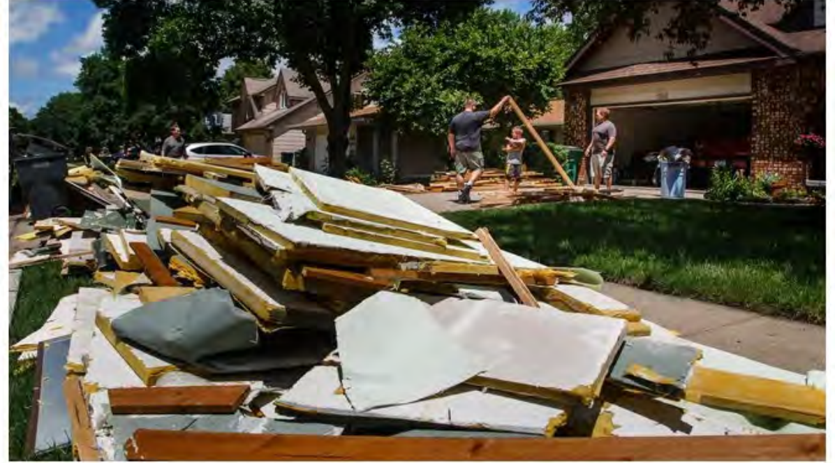
Steve Lucas of Waukee, right, helps sort through the wood he, brother Eric Bauer, left, and Bauer's son Austin, 7, center, tore out of their parents basement on Sunday, July 1, 2018, in Clive. They said there was about eight inches of water in the basement and everything needed to go.
